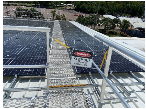
Photo 6.13– Area B West – Prohibited access to eastern sloping walkway from top walkway – Must have a Working at Height Permit approved by ADG Health & Safety Manager or approved delegate.
