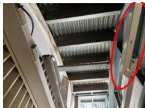
Photo 6.32 – Area Central PR filter – Guard rail open position
