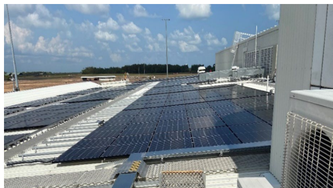
Photo 4.5 – Burn hazard and cut hazard – When walking & working near solar panels workers must wear gloves
