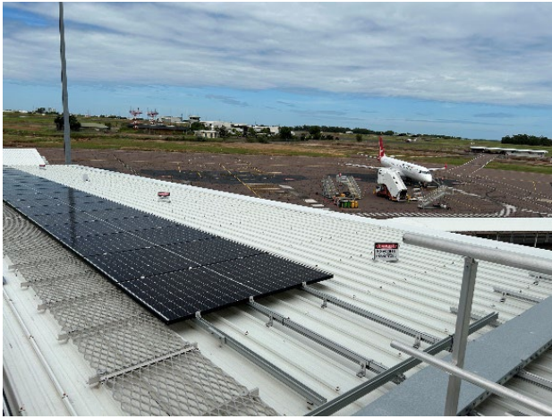
Photo 4.6 – Unprotected edges – No access outside designated walkway without a Working at Height Permit approved by the ADG Health & Safety Manager or approved delegate.
