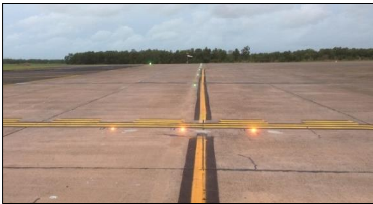
RWY Holding Position Lights
