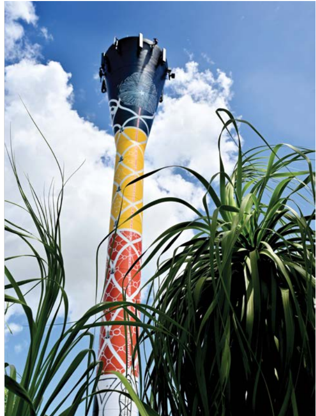
Communications equipment mounted to water tower.
