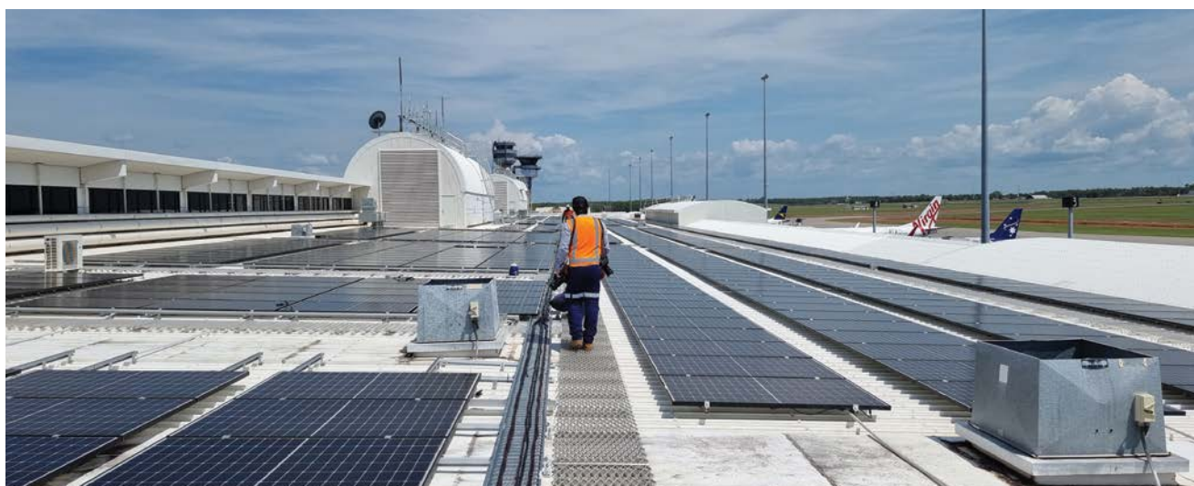
Rooftop solar array on terminal building
